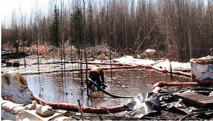
Enbridge clean-up of 63,000-gallon pinhole leak in Canada
