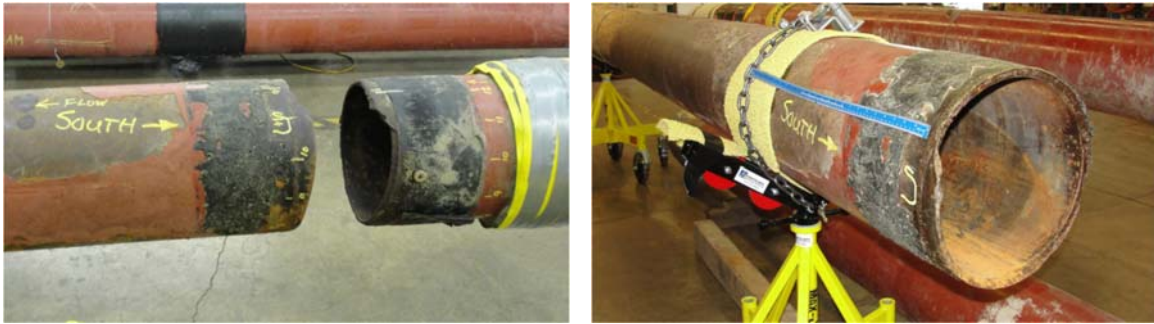
Guillotine rupture of ExxonMobil pipeline, Laurel, Montana, 2011 45
